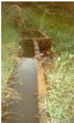
Another example of the problems with the civil works of the project where the forebay tank and channel have not been constructed properly
