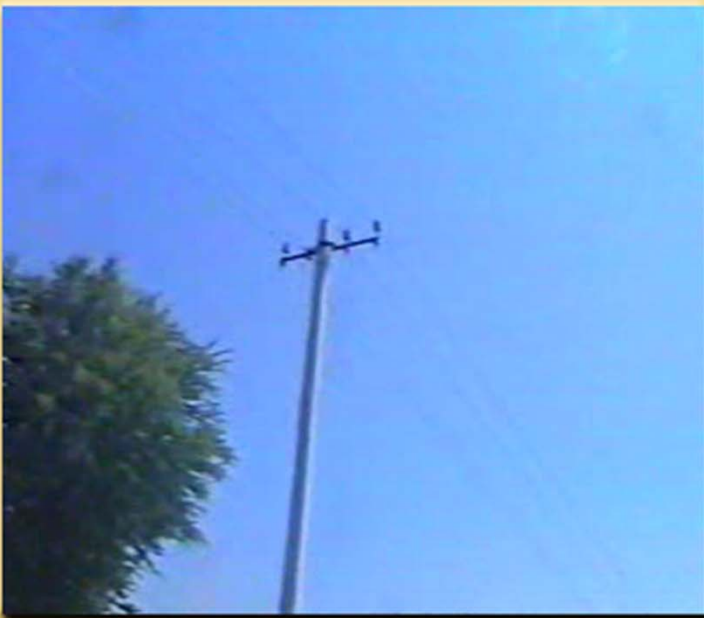
Existing LT 3Phase 4 wire line on support
