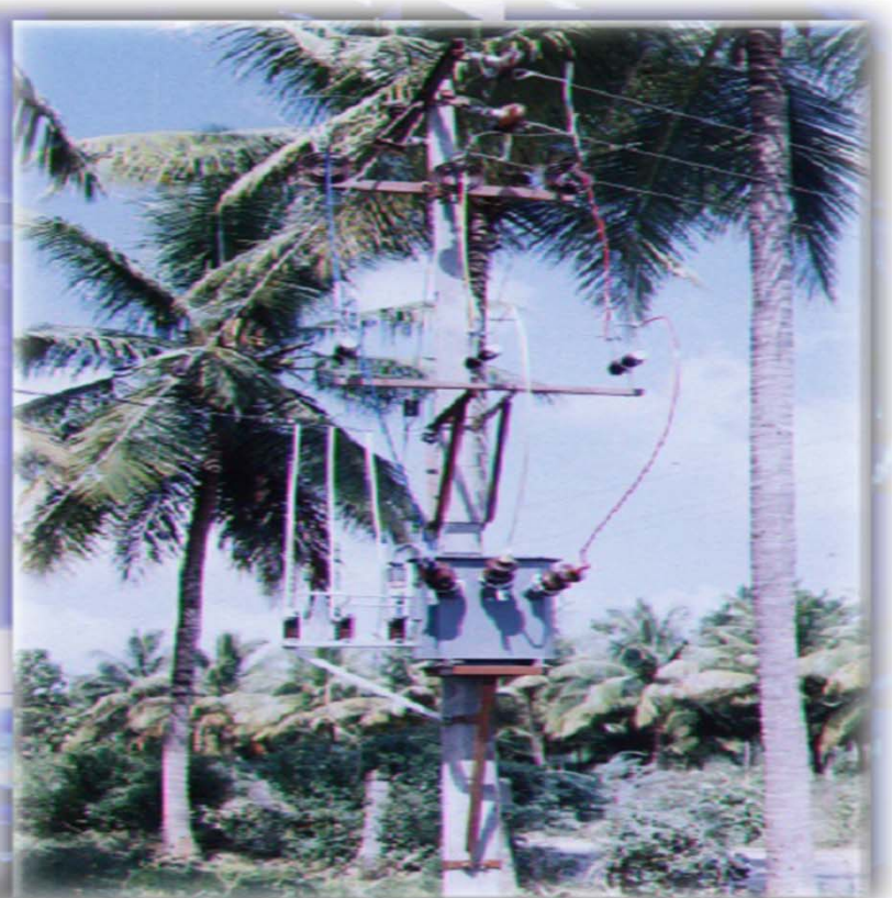
3ph 15KVA Dist. Transformer erected under HVDS to cater 2 to 3 services
