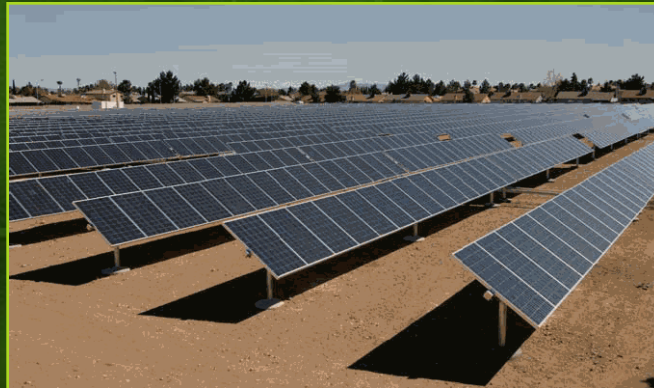
Solar PV Power Plant
