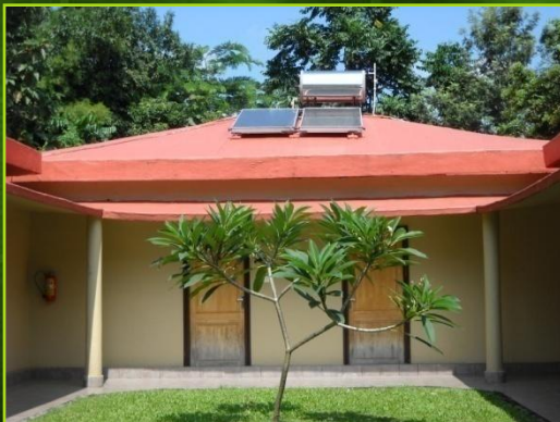
Solar Water Heater
