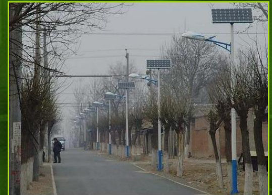
Solar Street Light
