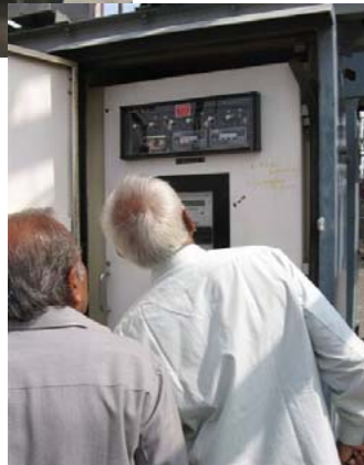
Meter reading at the feeder level.
