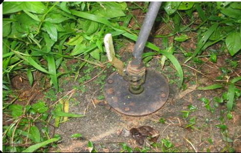
Biogas plant (gas outlet)
