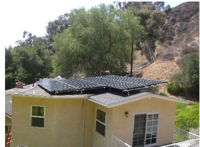
Photo: Pritesh Sampat, La Habra Heights Installer & Seller: AMECO, Long Beach, CA California Solar Initiative Funded System 2007, 8.2 kW
