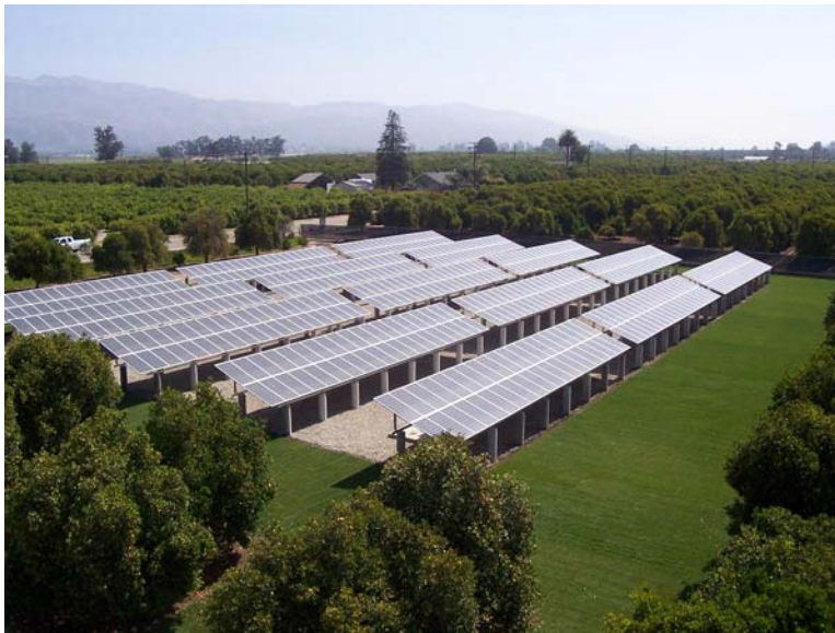
Photo: Travis Richardson, Hansen Trout Farm; Fillmore, CA. 105 kW California Solar Initiative Funded System, June 2007, Installer: GW Richardson Heating & Air Conditioning, Inc. Engineer/Designer: Kris Sutton, Travis Richardson
