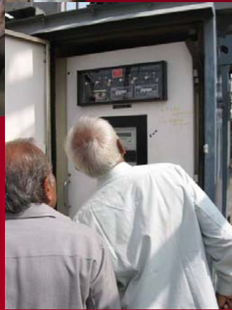
Meter reading at the feeder level.
