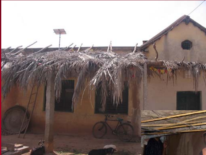
Solar panels atop the cocoon rearing centre
