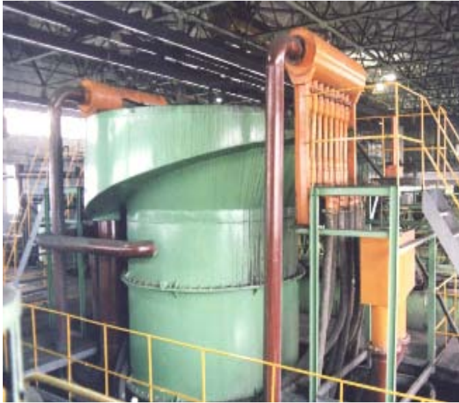
Column grade screening equipment
