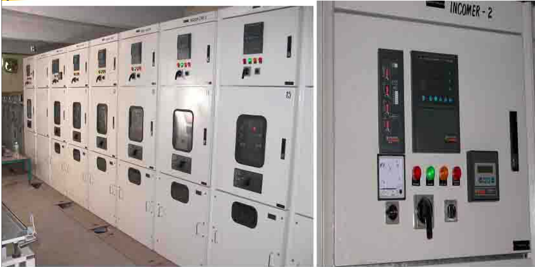
Newly Installed State of Art VCB
