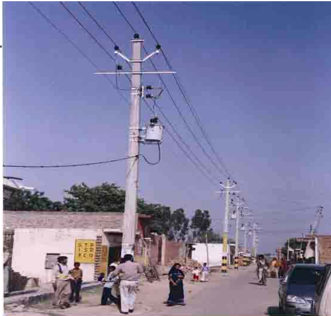
High Voltage Distribution System
